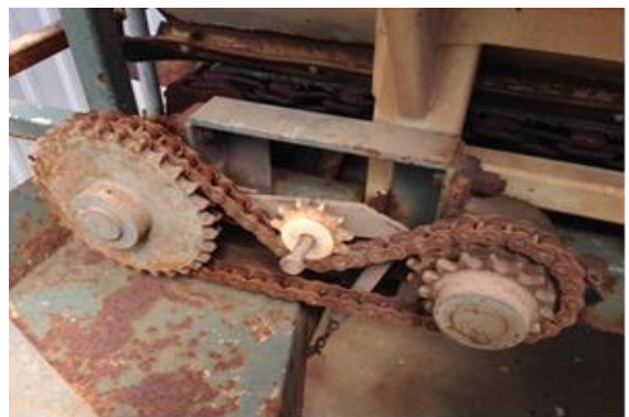
Chain guard missing
